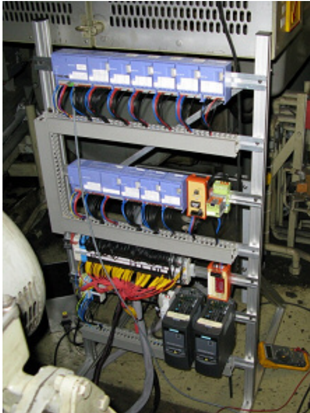
PLC and frequency converter on portable rack in the engine room
