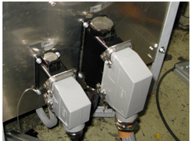
Raccordement automate programmable - locomotive
